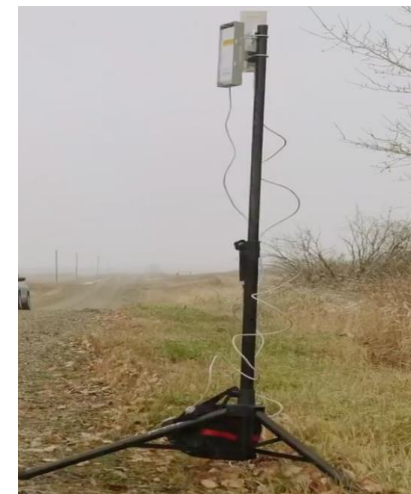
Temporary installation on a Tripod
